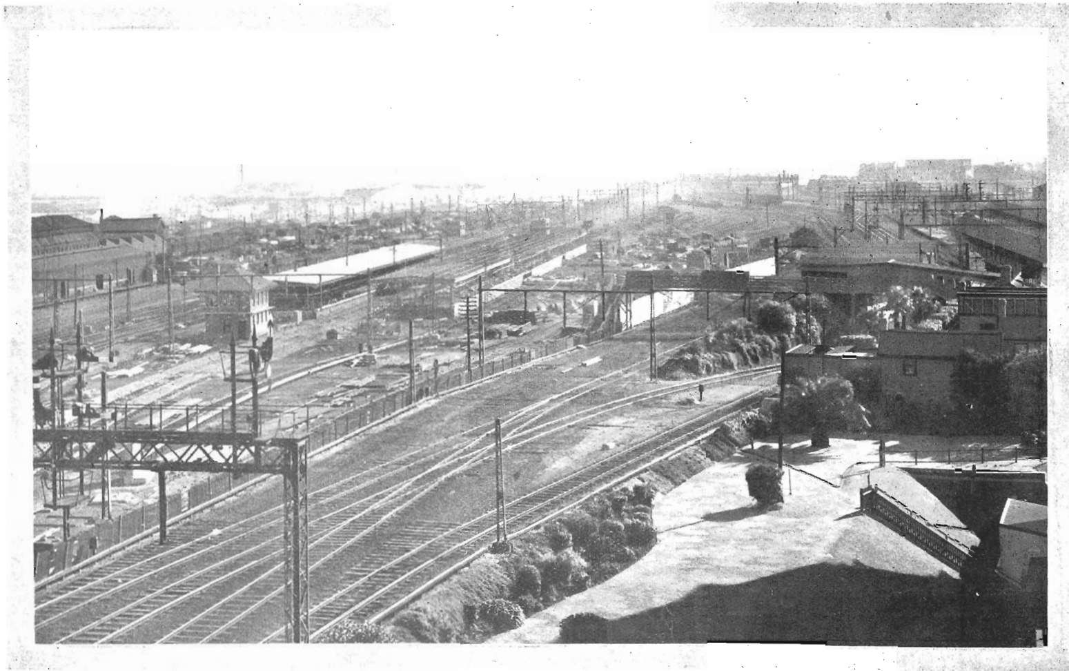
New Island Platforms to accommodate Suburban passenger traffic are in course of erection. Extensive re arrangement of tracks is also being effected.
